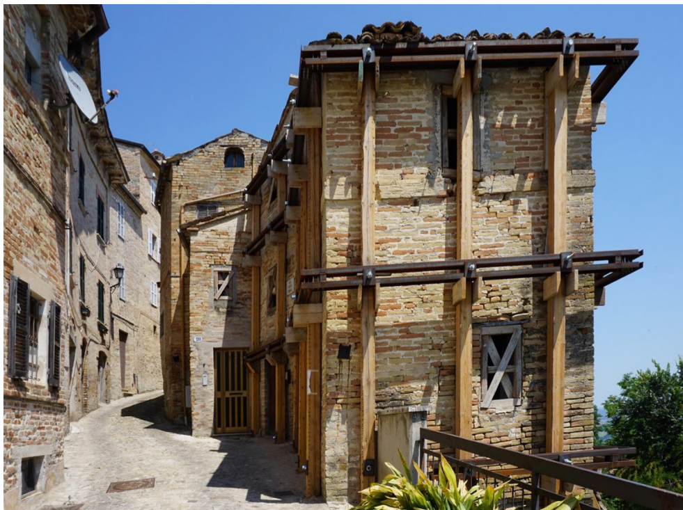
Figure 5. Reinforced buildings in Falerone after the earthquake, Váli, I., (2017)
