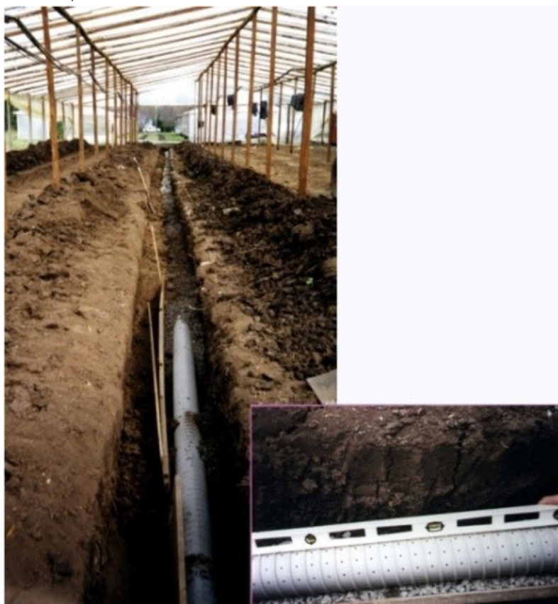
Figure 8. PVC drains installed on top of the Btss horizon covered with granite stone and detail of the drain with use of level to maintain slope
